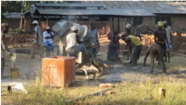
In July, workers started building the dining and assembly hall at Tumaini Lutheran Seminary in Tanzania.
