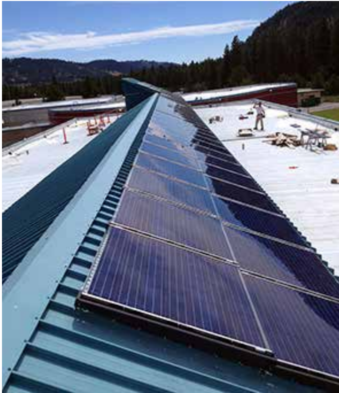
Solar panels on the middle school produce enough electricity for three homes
